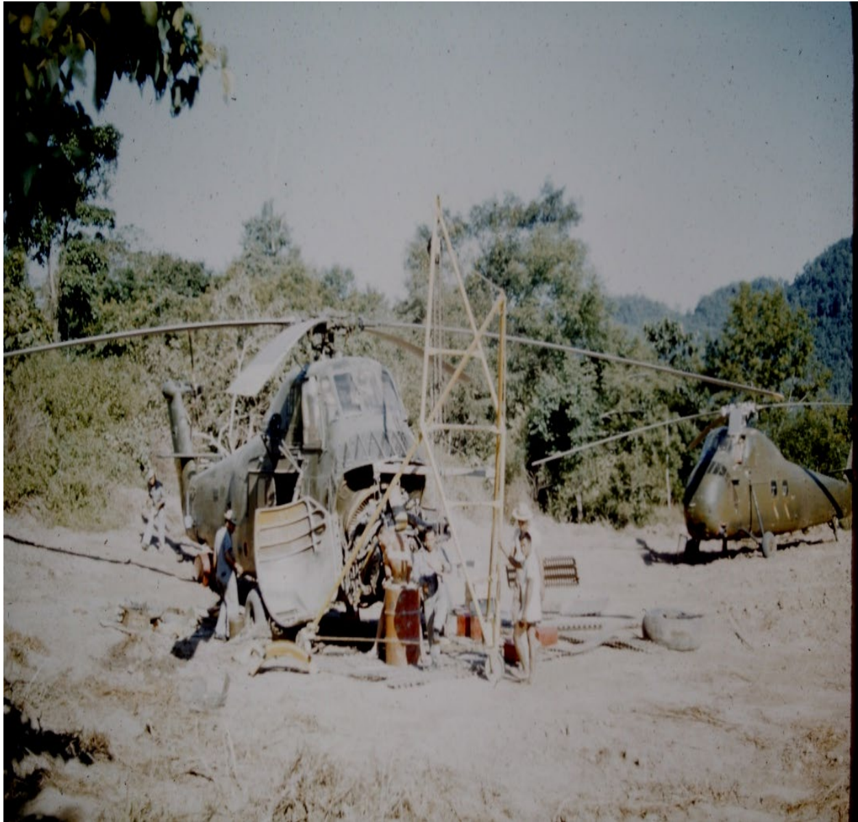
Front view of Hotel Romeo with the intricate "field expedient" wooden lifting device erected to remove and install the R-1820 engines. Ron Clarke's H-34 to the right. Ron had delivered supplies to the site. Clarke Collection.
