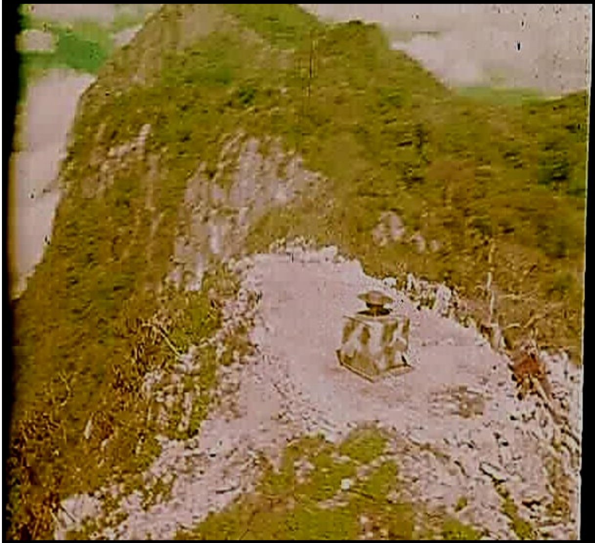
The TACAN unit emplaced at the designated site on top of Pha Thi following Chinook helicopter sling load delivery.
